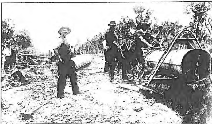
Laying pipes in the ranges between Mundaring and Bakers Hill. Note expander and trolley in pipe.
