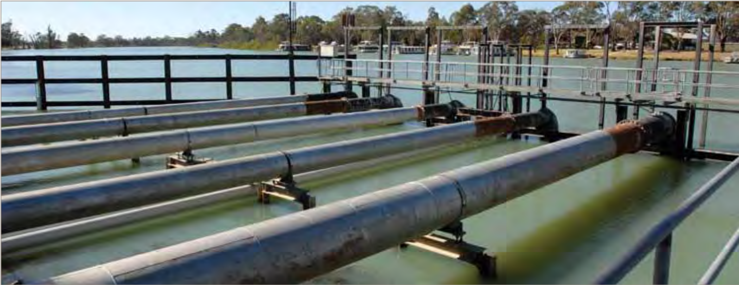
Irrigation pump station on the River Murray near Berri, South Australia
