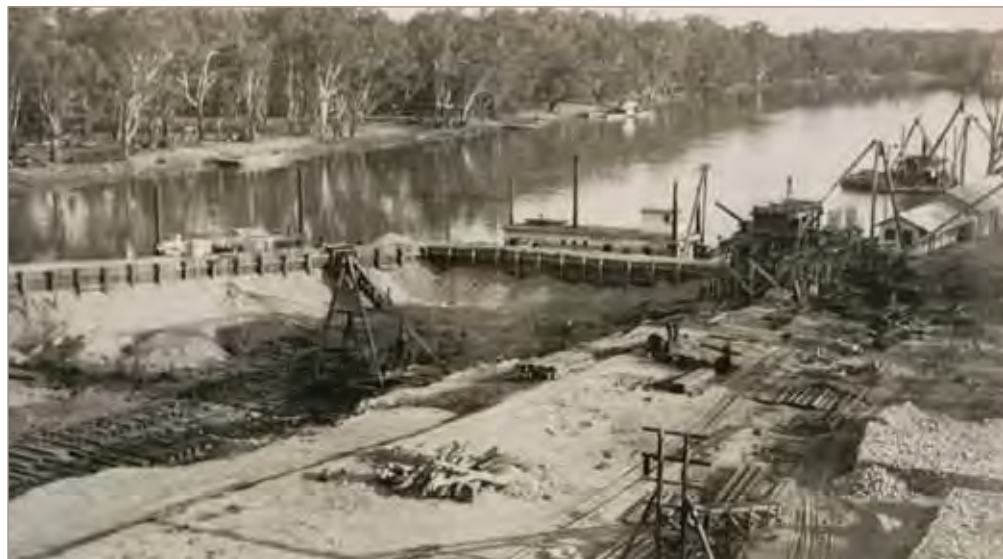
Construction of Lock 8 on the River Murray west of Wentworth, 1935, New South Wales
