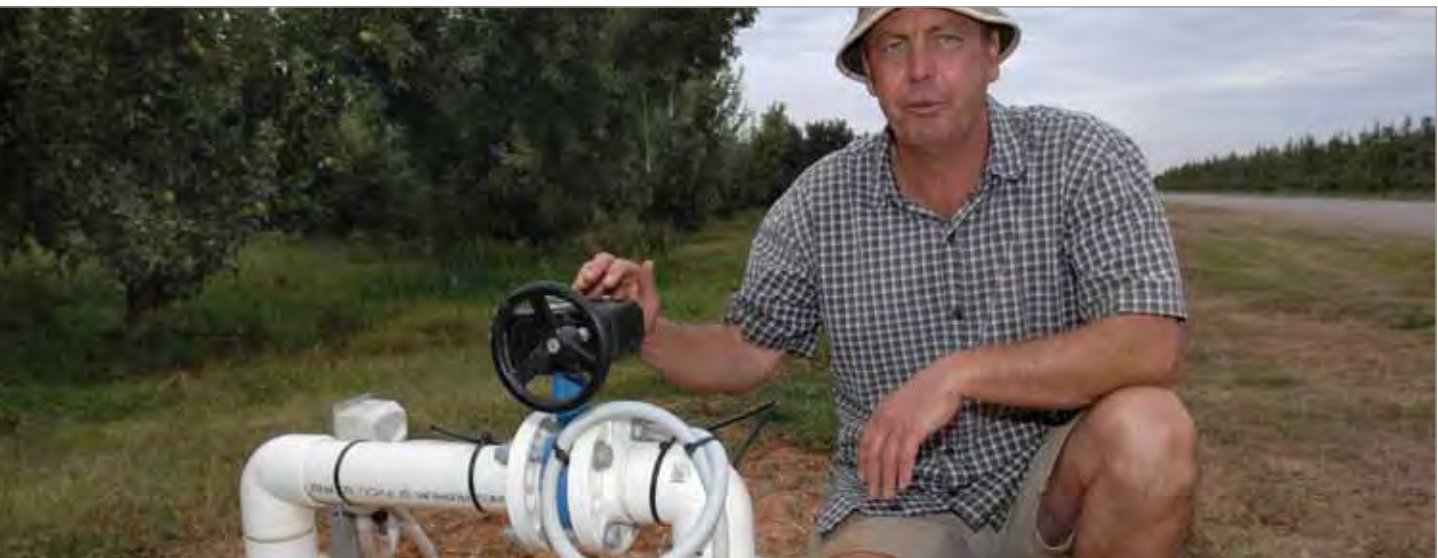
Bore used to supplement the water supply at an orchard near Cobram, Victoria
