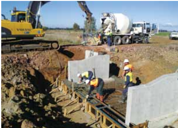
Regulator installation near Wright Road, Leeton.
