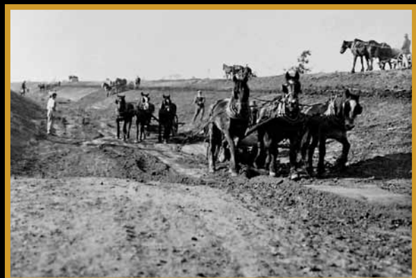
Construction of the Main Canal (between Beelbangera and Penfold's Bridge near Griffith) c.1915.
